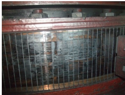
Example of commutator with presence of significant ridges and flat spots
